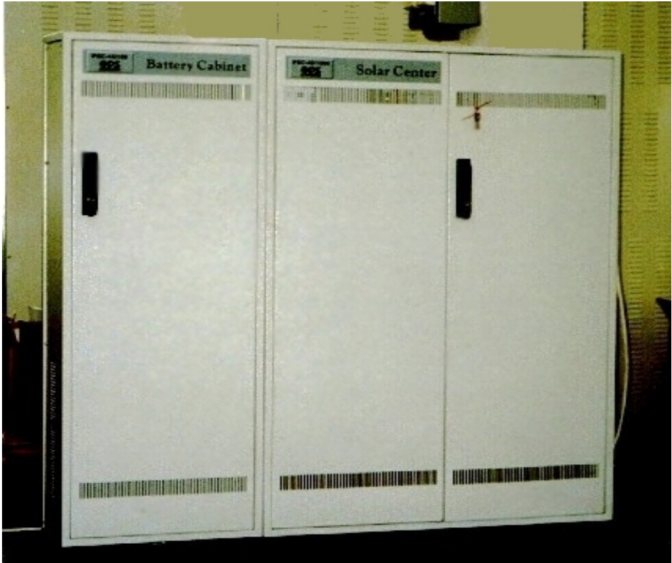
Powerstar PSC-48V/3500 complete photovoltaic solar system with battery cabinet
